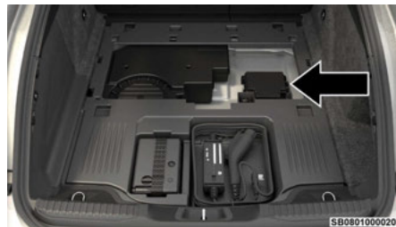
Rear Power Distribution Center
