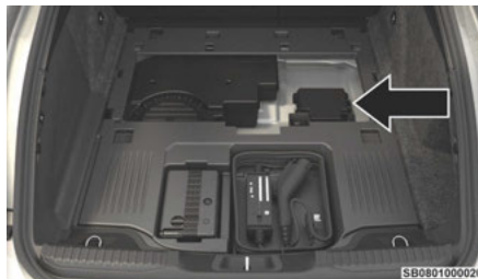
Rear Power Distribution Center
