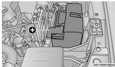
Positive (+) Battery Post
